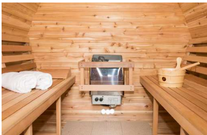
Inlet under electric heater on Back wall
