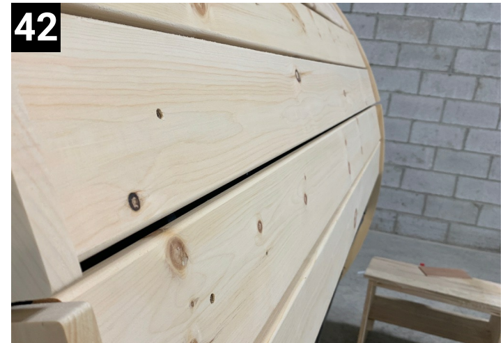
42 About 1/4" spacing between roof boards
