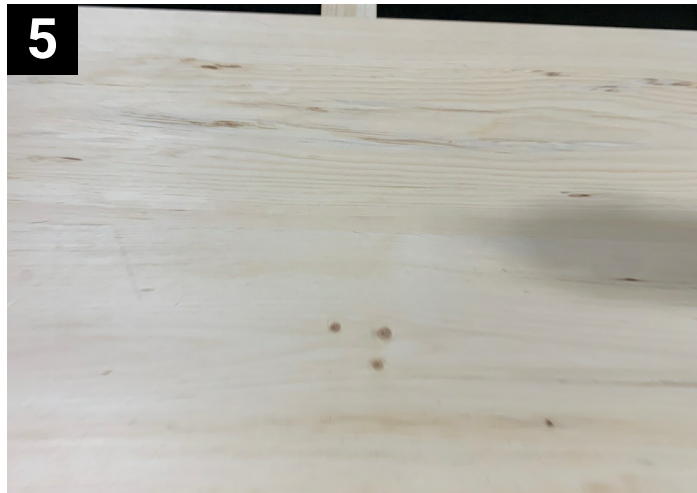
5 No screws in Center isle way.
