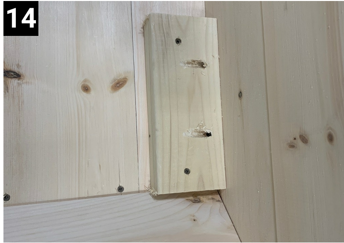
14 Screw down floor cleats then push down on wall board so it's tight to floor then put in the 2 pocket screws.
